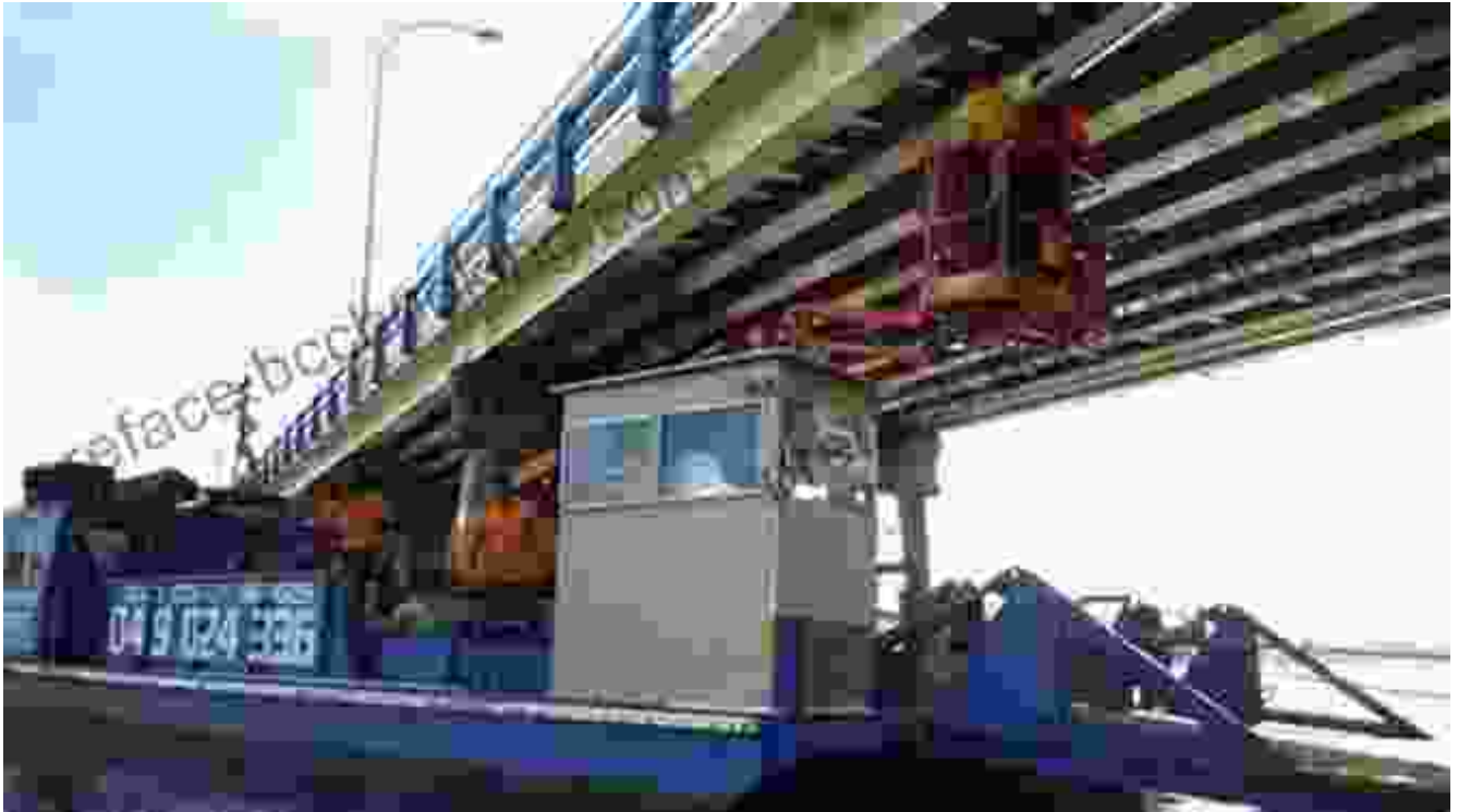
A cherry picker being used to inspect a bridge for structural integrity.
