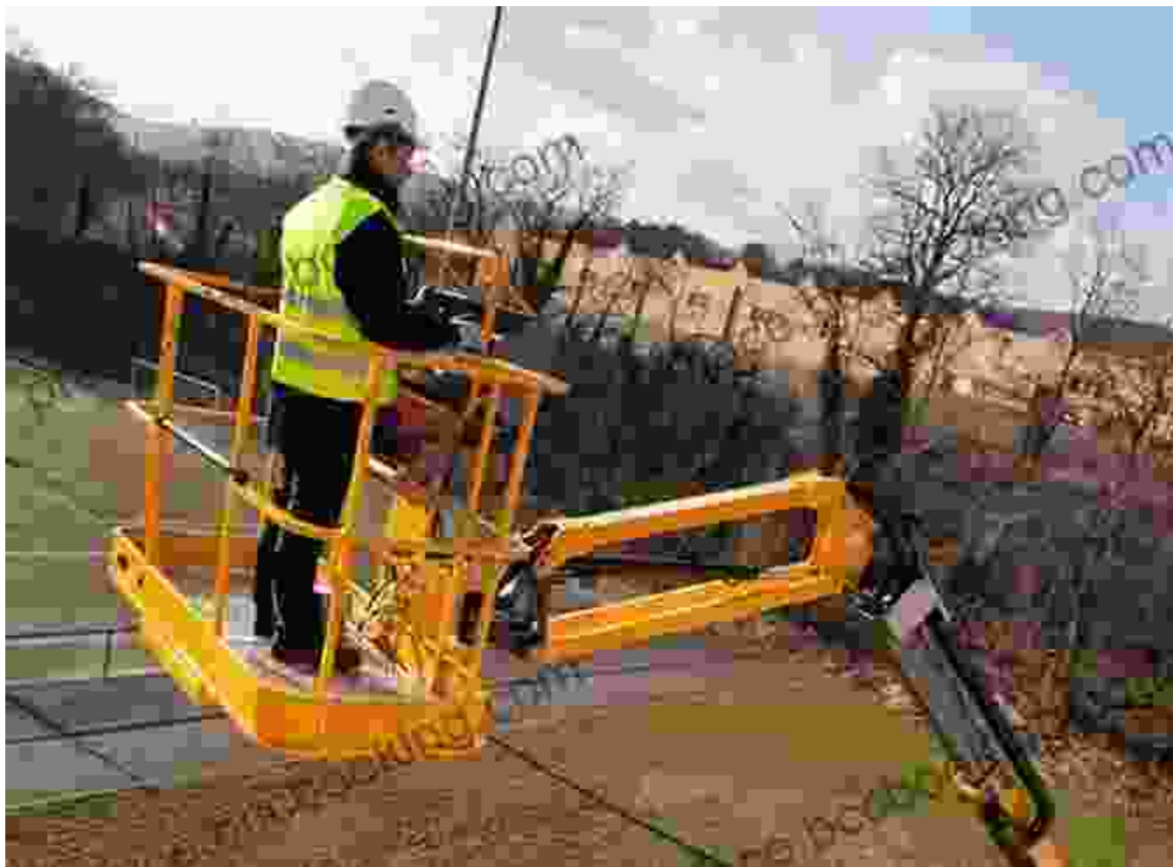
A cherry picker being used to install roofing on a new building.
